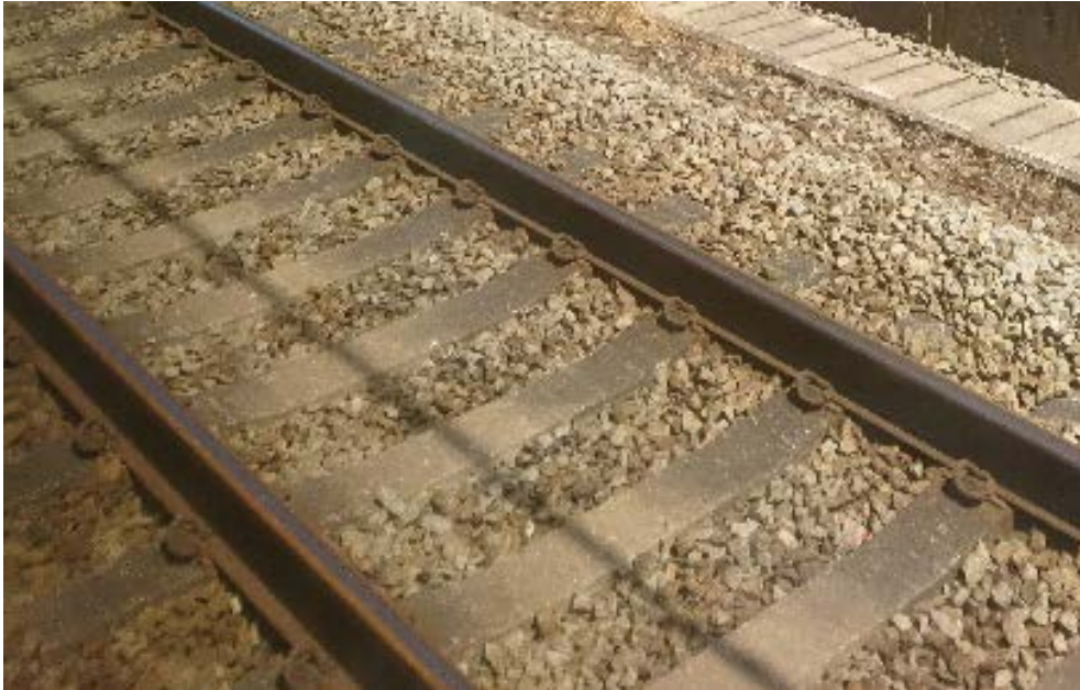
Figure 2: Ballast layer is contaminated by upward clay migration
