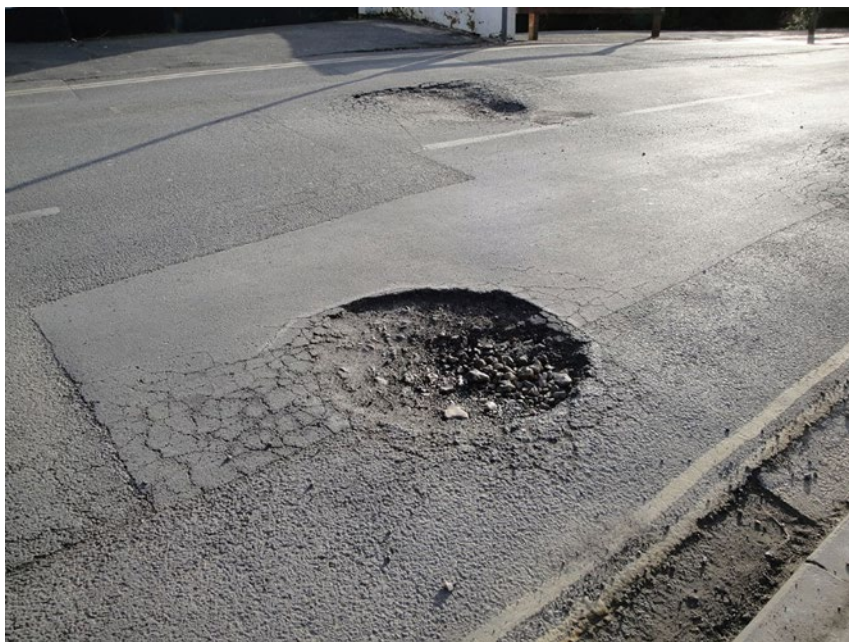
Figure 3: Potholes on asphalt pavement
